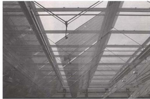
Detail of the movable louvers for natural lighting and natural ventilation of the atrium ceiling
